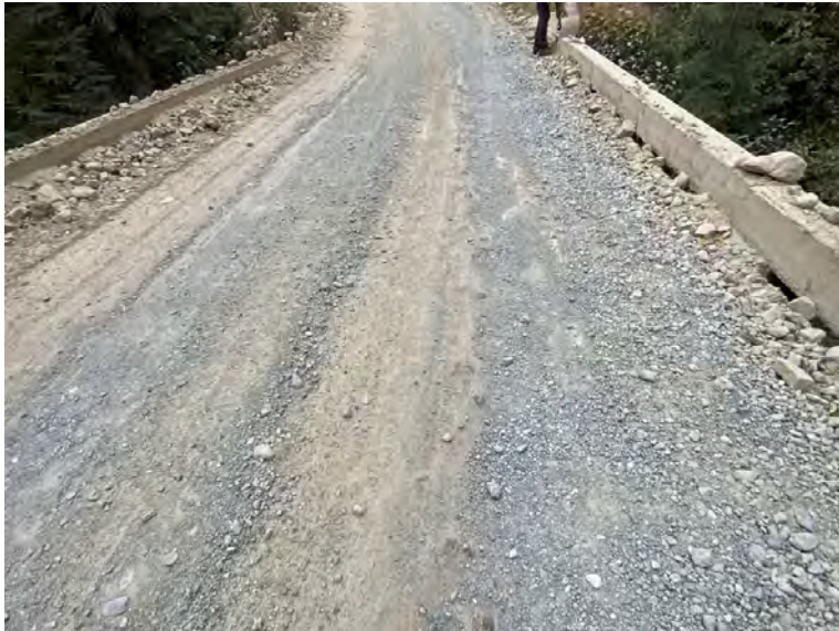
Worn running deck
